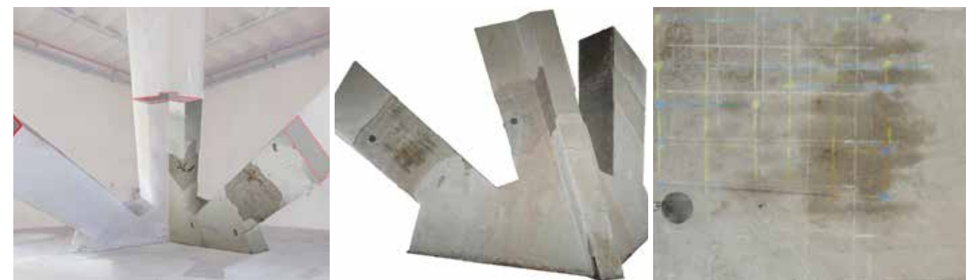
3a 9.5: Texturized model of the base of the arches, enabling corings, cracks and exposed iron to be located, and the positions of the sensors used during diagnostic investigations. Below: an example of orthophoto of a recognition area of the column reinforcement grid.
