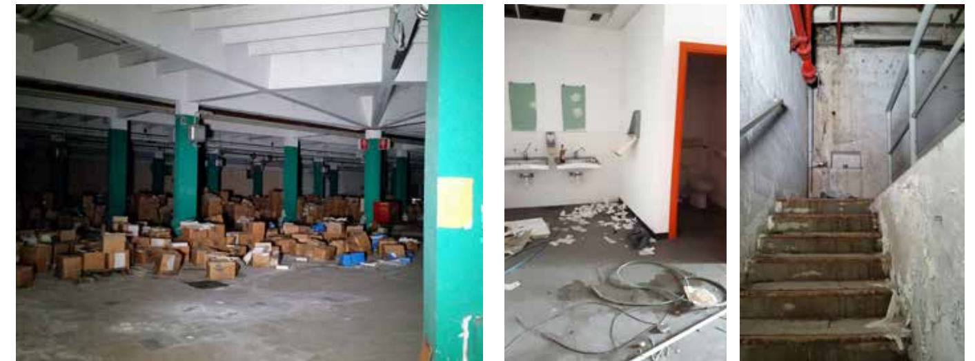
3a 3.4. a, b, c: For underground environments, it was necessary to use traditional 3D scans, but in general, all the service areas and stairs were detected by means of mobile scans from hand-held scanners.
