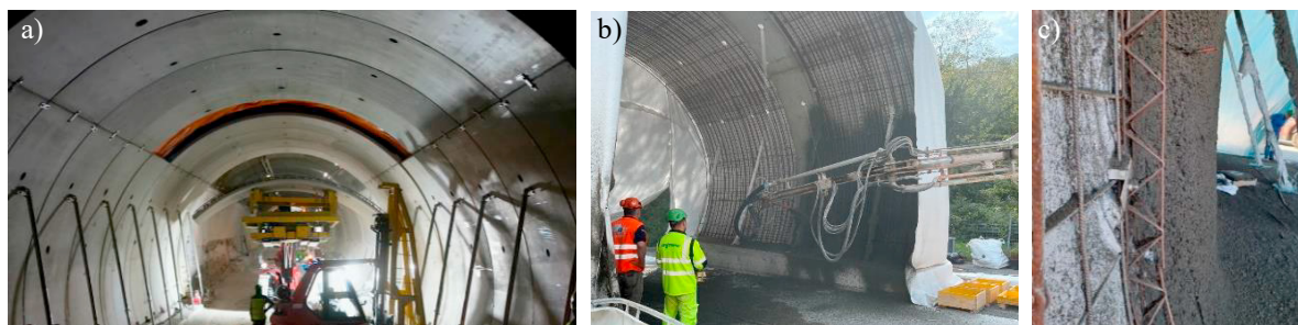
Fig. 7 a) “Colle Marino” tunnel construction site – relining by high strength shotcrete b) and c) “San Fermo” tunnel - Field test of shotcrete application
