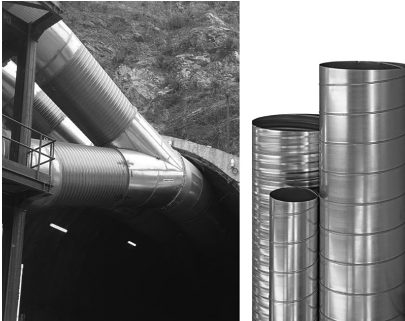
Figure 6.53 One application of rigid ducts and classical typologies.
