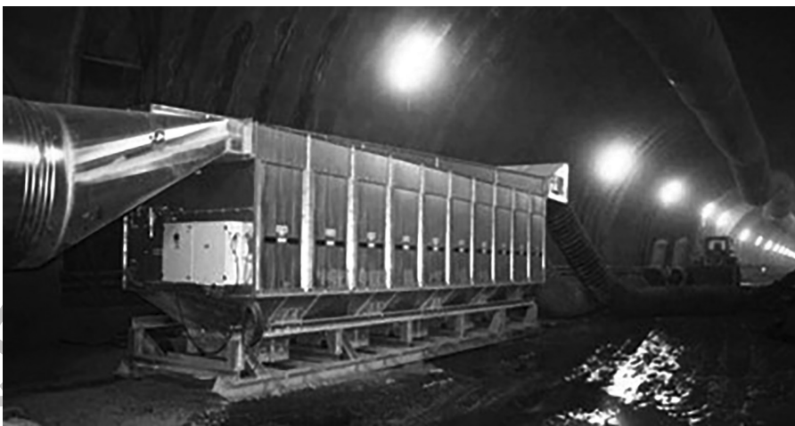
Figure 6.59 Mixed ventilation system with de-duster equipment and its suction spiral duct.
