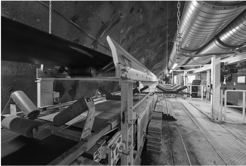
Figure 6.8 TBM backup extension station. (Courtesy of Marti Technik.)
