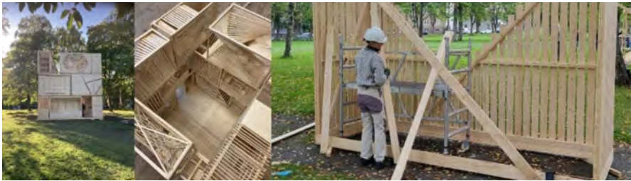
Fig. 6. Full scale building by 1st year students in Trondheim, 2023 (Photos by A. Gilberg and Z. Živanović, NTNU.)
