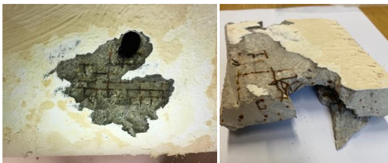
Figure 2: (a) Surface scarification of the ferrocement element before the extraction of the sample. It is possible to see the detachments of the painted surface due to possible water infiltrations. (b) Collected sample of ferrocement. It is possible to see the various layers of wire mesh and their state of conservation.
