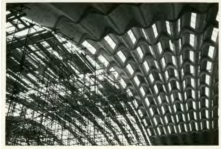
Fig. 4. This photo of the construction site shows the mobile scaffolding system used to build the vault (Archivio Privato Ravelli).
