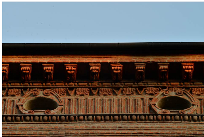
Fig. 3. Upper cornice of the 17 th century façade: replacement and partial consolidation of the closing courses and some decorated corbels can be appreciated. In this case, the moulded terracotta elements that make up the corbels, which are the most fragile part of the system, are adequately protected by the upper part of the cornice, which is made of solid bricks with a traditional masonry texture (Pictures were taken on February 2024, by M. Zerbinatti).
