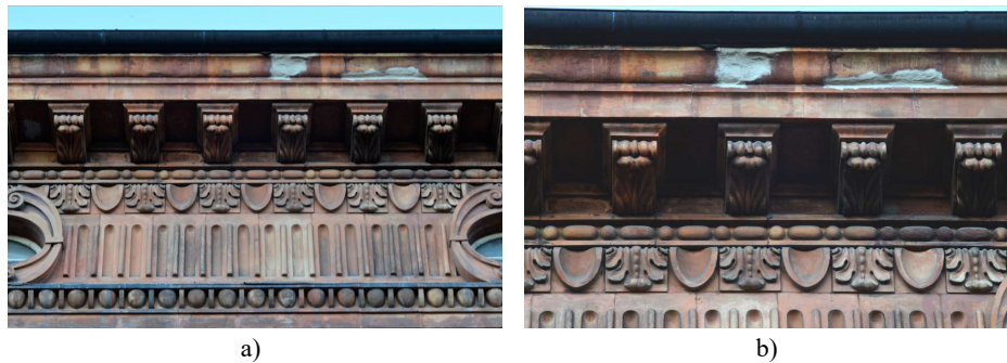
Fig. 2. a) The overall view of a module of the decorative apparatus of the crowning cornice of the 19 th century façade: noteworthy is the design of the cornice above the corbels, which is no longer made with repeated courses of solid brick elements, but with the superimposition of two specially shaped elements made on a bench; b) Detail of the upper cornice of the 19 th century façade. Recent cleaning work has revealed earlier additions and consolidations to the hollow brick mouldings that complete the decorative system. The deterioration of these elements is closely linked to the presence of persistent infiltration from the rainwater collection system. (Pictures were taken on February 2024, by M. Zerbinatti).
