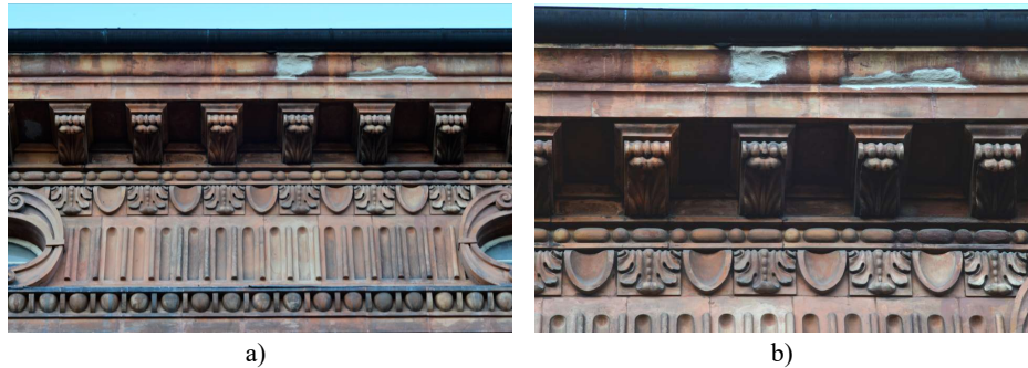
Fig. 2. a) The overall view of a module of the decorative apparatus of the crowning cornice of the 19 th century façade: noteworthy is the design of the cornice above the corbels, which is no longer made with repeated courses of solid brick elements, but with the superimposition of two specially shaped elements made on a bench; b) Detail of the upper cornice of the 19 th century façade. Recent cleaning work has revealed earlier additions and consolidations to the hollow brick mouldings that complete the decorative system. The deterioration of these elements is closely linked to the presence of persistent infiltration from the rainwater collection system. (Pictures were taken on February 2024, by M. Zerbinatti).
