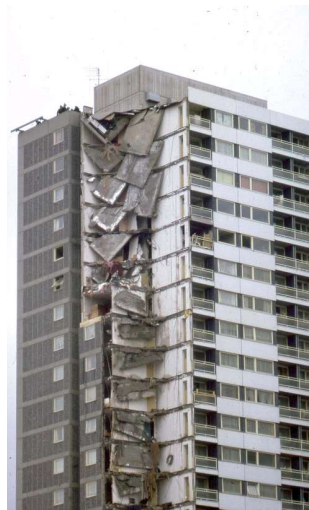
Figure 1.1 Ronan Point Building collapse, May 16 th 1968, London (UK).
