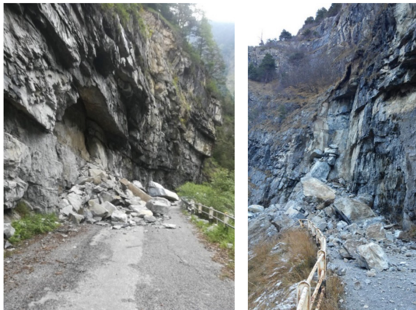
Figure 1. Two views of road sections extensively affected by severe rockfall events.
