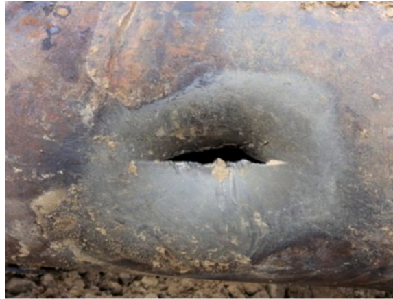
Fig. 2. Typical excavator puncture on pipe surface.
