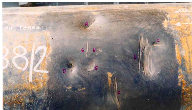
Fig. 1. Pipe portion with dents (marked with letters A, C, D), gauges (E, F, G), and combination of both (B).
