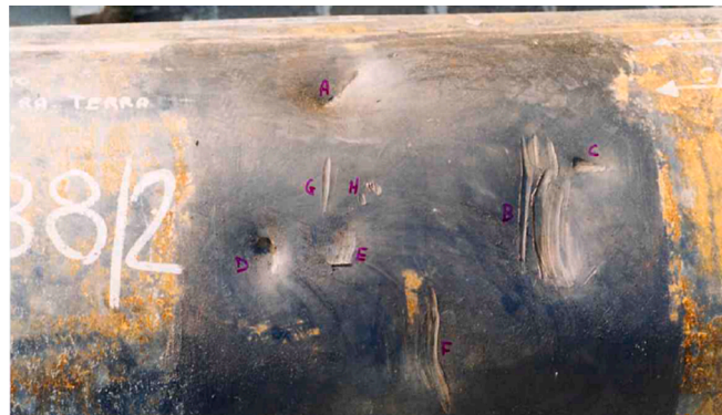
Fig. 1. Pipe portion with dents (marked with letters A, C, D), gauges (E, F, G), and combination of both (B).
