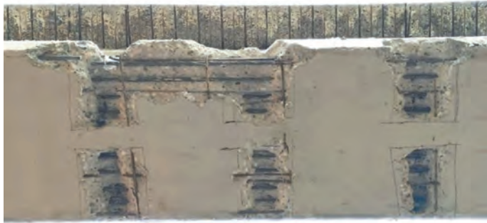
Figure 3. Strands cutting in B5-P46/47 girder (bottom view).
