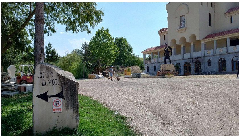
Figure 12: At the construction site of the new church. The stone indicates the way to the spring. Photograph by Giuseppe Tateo.
