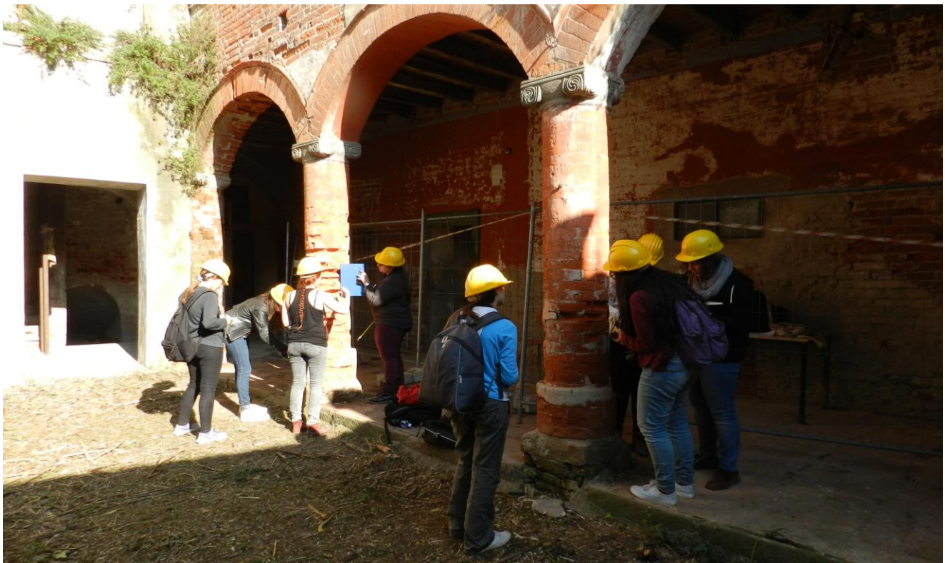
Fig. 6: Pinerolo, the so-called Palazzo dei Principi d'Acacia, seen from the court. Students engaged in activities to assess the state of preservation of brick columns (M. Mattone 2016).
