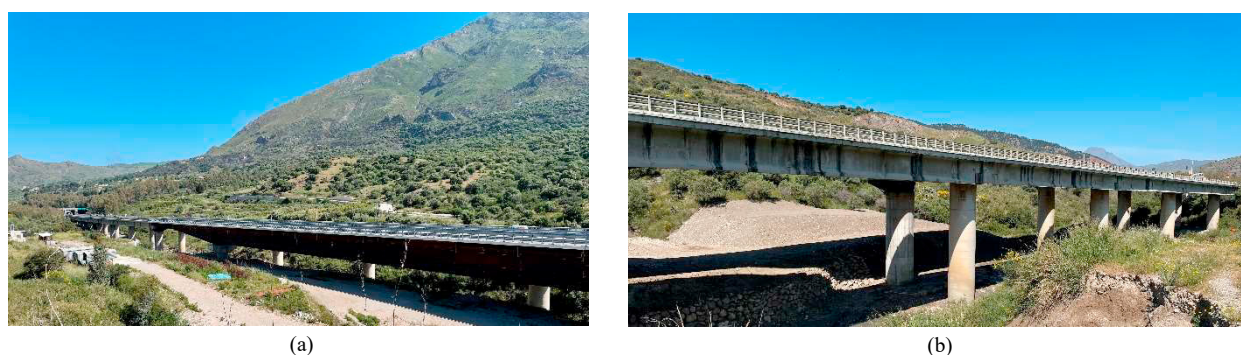
Fig. 2 Viadotto Imera I: (a) Right desk, steel construction after collapse; (b) Left desk, pre-stressed reinforced concrete
