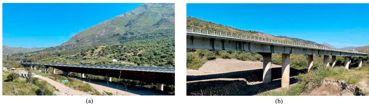
Fig. 2 Viadotto Imera I: (a) Right desk, steel construction after collapse; (b) Left desk, pre-stressed reinforced concrete
