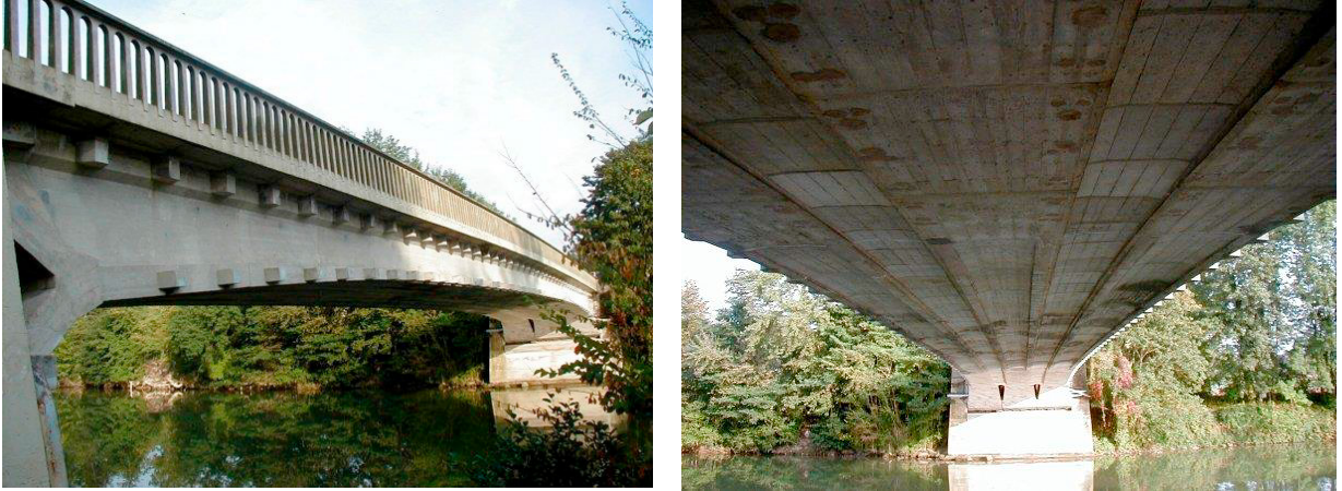
Figure 2 (a & b) Views of the Luzancy Bridge by E. Freyssinet 1946 (Courtesy of www.structurae.net ).
