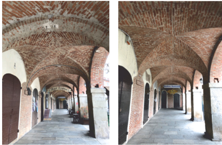
Fig. 2. View of two different 18th century vaults of the portico, with radial masonry pattern (right) and diagonal pattern (left).
