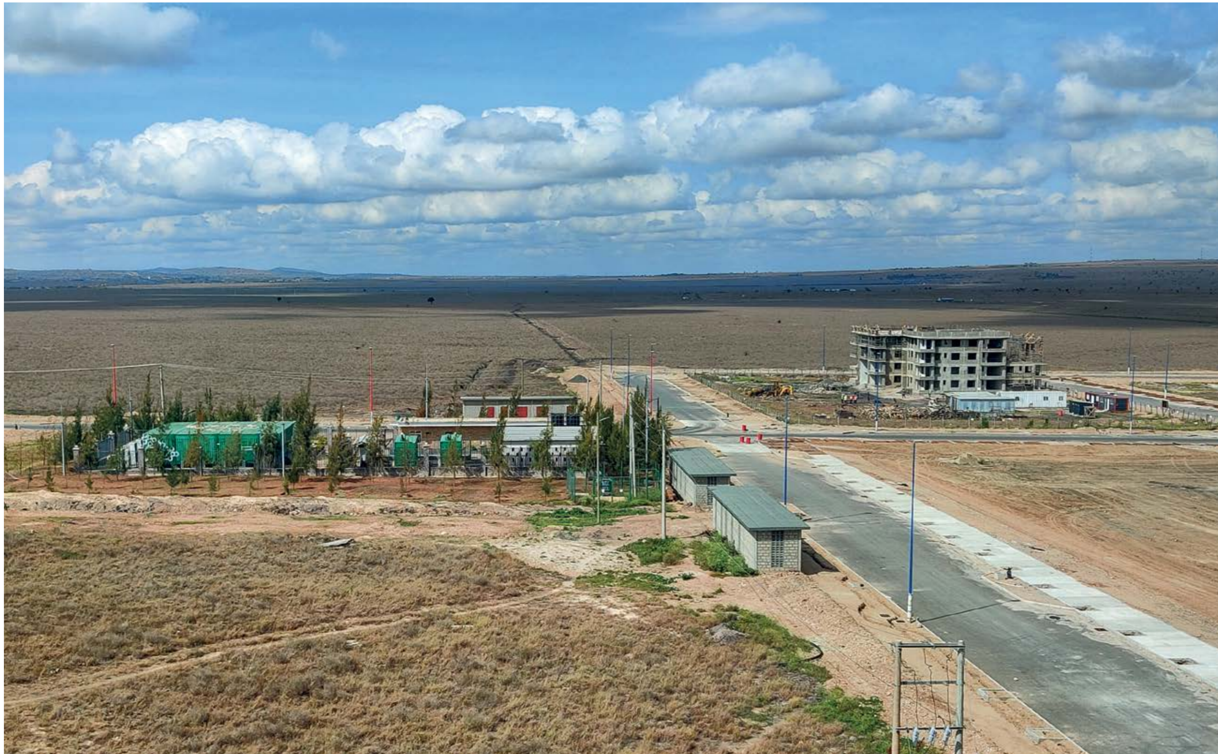
Fig. 1 | The construction site of Kenya's national data centre, funded by a Chinese loan and delivered by Huawei (credit: Andrea Pollio - China Room).
