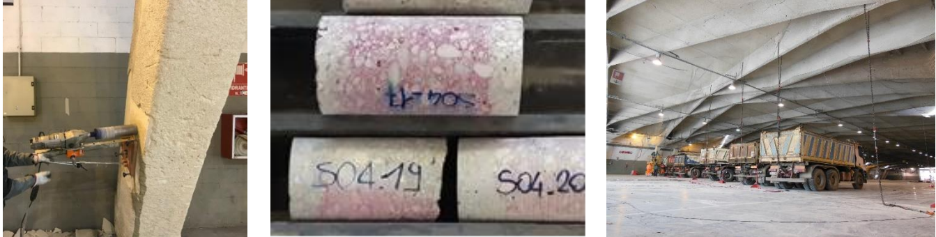
Figure 7 Pavilion V: Extraction of a concrete sample from a longer strut beam (left); carbonation tests on the samples of the ribs (center); view of the static tests with trucks connected to the ribs through jacks (right) [34].
