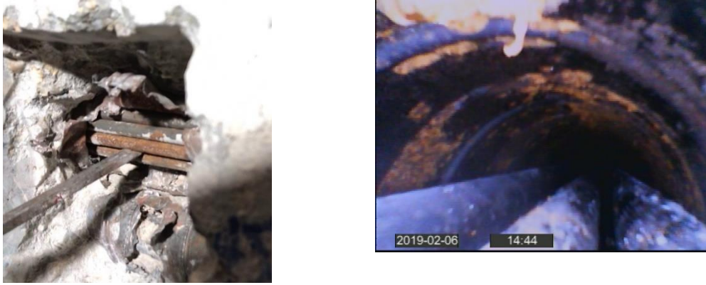
Figure 11 Visual inspection of post-tensioning tendons in the ribs at location S07.01 (left), and endoscopy inspection inside a duct of the rib at location S07.02, where grout filling of the duct is seen to be incomplete (right) [34].
