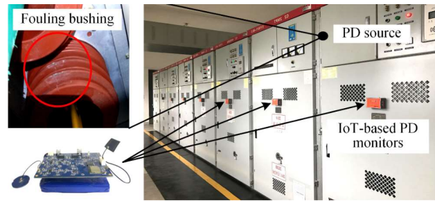
Fig. 13. Online PD monitoring of MV switchgears via IoT-based PD monitors.
