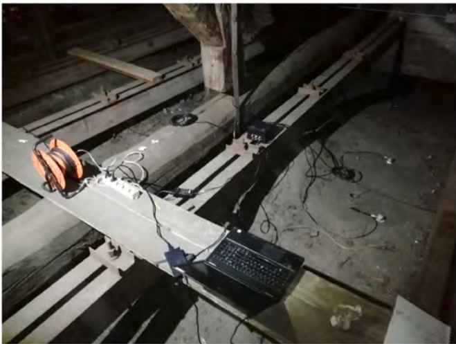
Fig. 6. AEmission System: Multi-channel acquisition system and sensors applied to the vault extrados.
