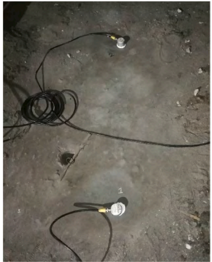
Fig. 7. Two of the eight sensors, positioned on the extrados of the central nave vault.
