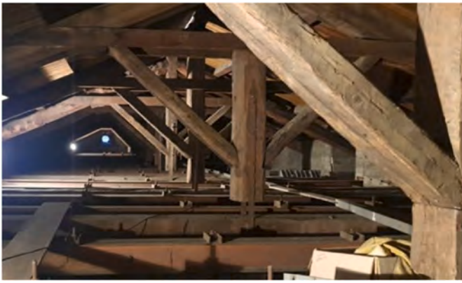
Fig. 4. Overall photo of the wooden trusses in the attic of the central nave.
