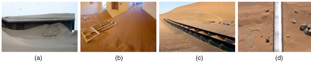
Fig. 1. Windblown sand effects on structures and infrastructures: (a) buried houses in Waldport, Oregon; (b) in In-Salah, Algeria; (c) buried railway track in Namibia; and (d) rail deformation. [Reprinted (a–c) from Engineering Structures , Vol. 178, L. Raffaele and L. Bruno, “Windblown sand action on civil structures: Definition and probabilistic modelling,” pp. 88–101, © 2019, with permission from Elsevier; reprinted (d) from Journal of Wind Engineering and Industrial Aerodynamics , Vol. 177, L. Bruno, M. Horvat, and L. Raffaele, “Windblown sand along railway infrastructures: A review of challenges and mitigation measures,” pp. 340–365, © 2018, with permission from Elsevier.]
