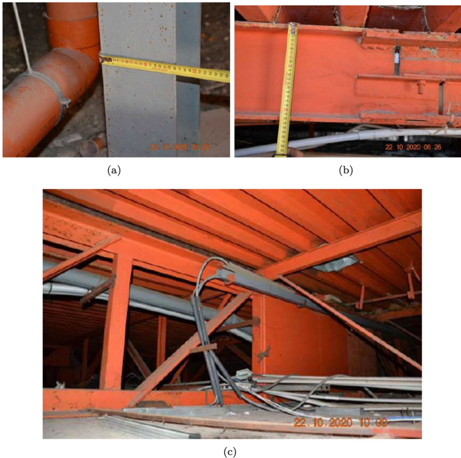
Fig. 4 a HEA160 short column supporting the raised floor; b detail of a hinged connection at the raised floor level; c close-up of a rigid connection on the primary truss beams
