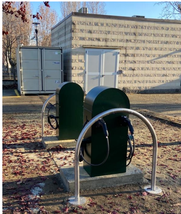
Figure 3. Caio Mario substation and low-power chargers inspired by Turin's iconic "Turèt" fountains [30].
