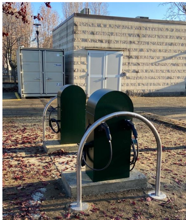
Figure 3. Caio Mario substation and low-power chargers inspired by Turin's iconic "Turèt" fountains [30].
