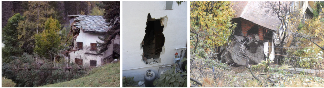
Fig. 3. Damaged buildings due to rockfall events. Photos by courtesy of Autonomous Region of Valle d'Aosta and ARPA Piemonte.
