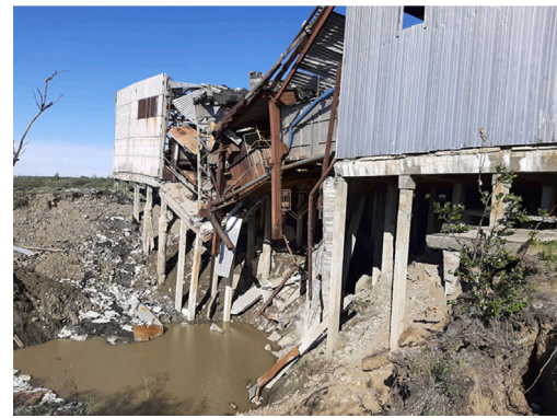
Fig. 2. Partial collapse of a building in Chersky, North-Yakutia, Russia due to permafrost thawing [39].
