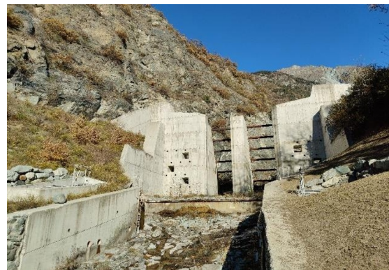
Fig. 1 Example of filter barrier, Saint-Vincent, Aosta Valley (Italy)
