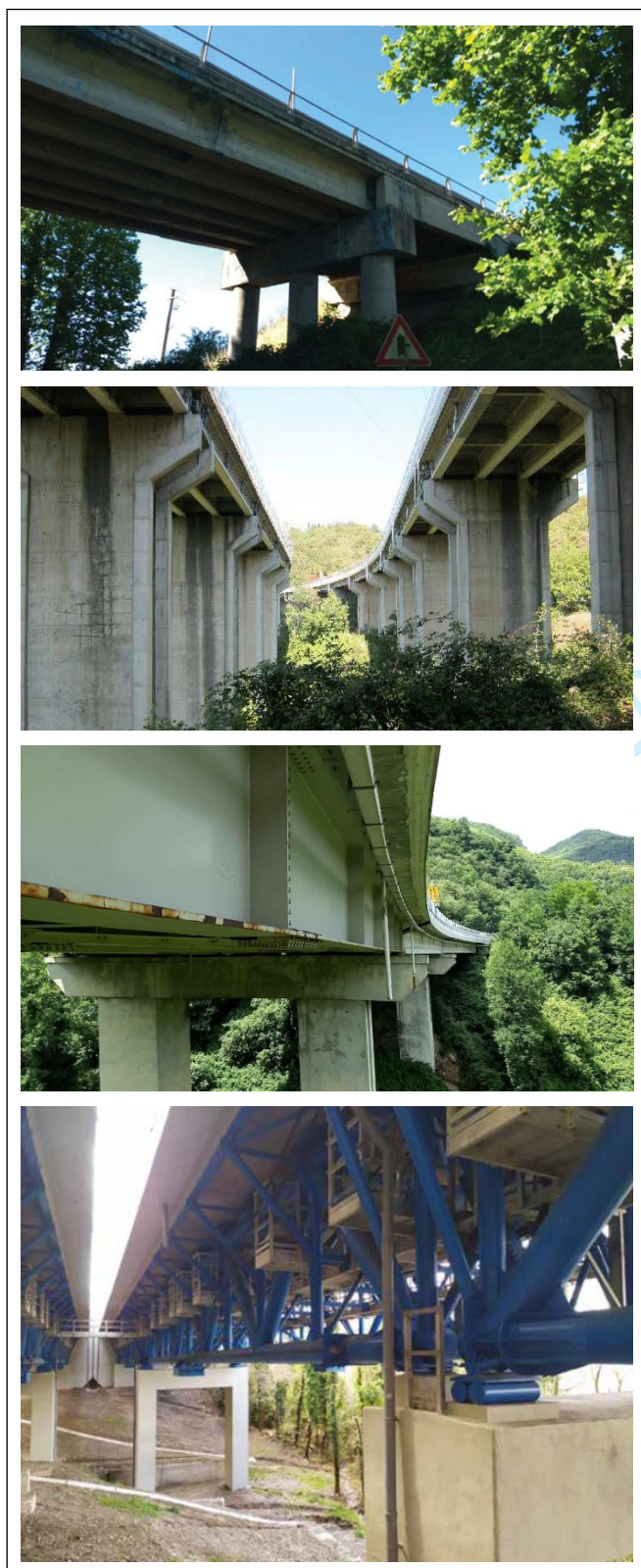
Figure 1 Some cases of bridges assessed by ASPI with the external review by Politecnico di Torino.
