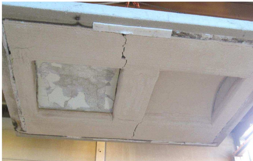
Figure 38 - (a) Failure between the intrados of V.04.c and the top of the confinement wall; (b) Intrados view of V.04.c and V.05.c after the fire test.
