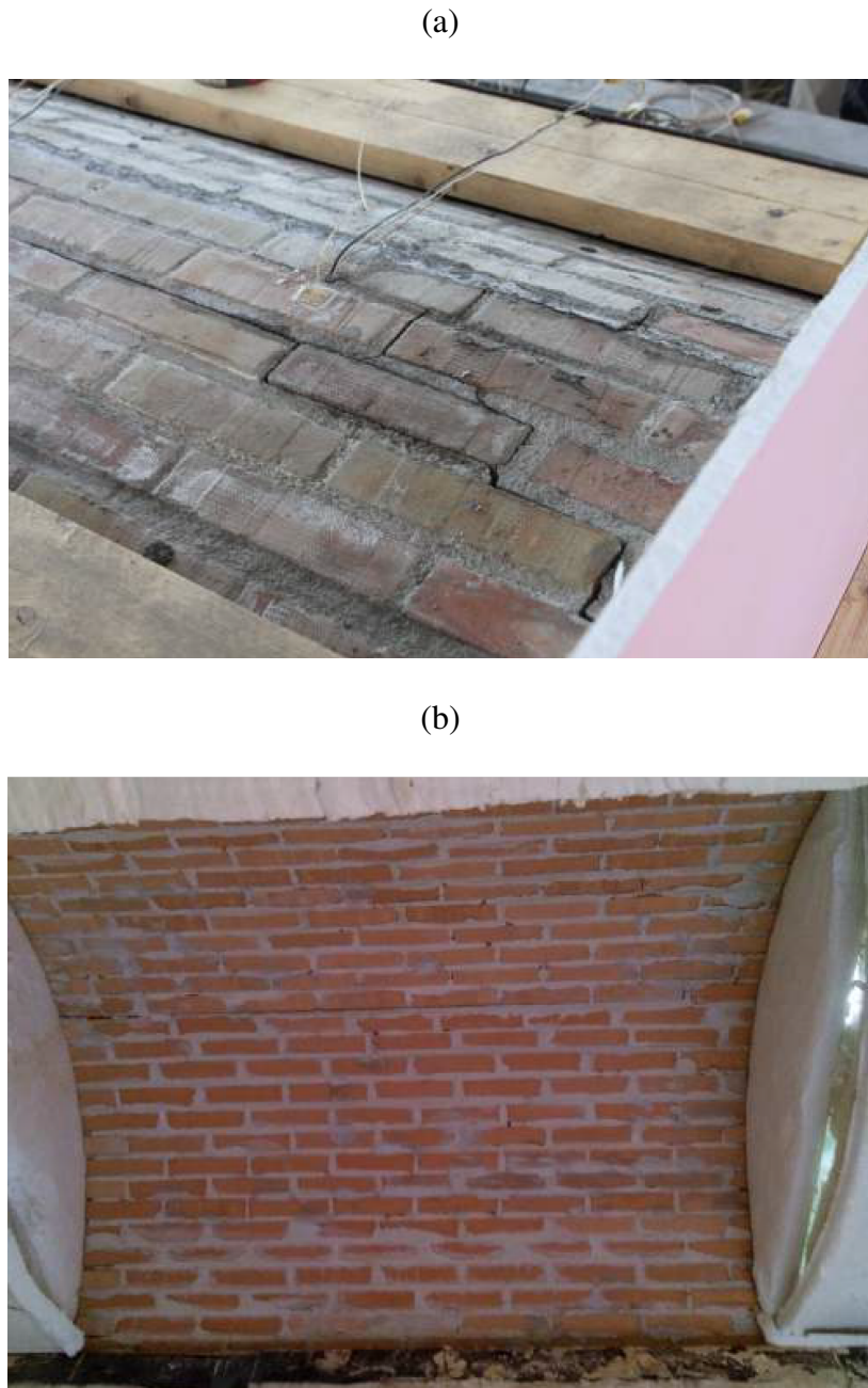
Figure 30 - V.03.u : (a) crack pattern in the midspan (extrados view); (b) internal view of the vault after the fire test
