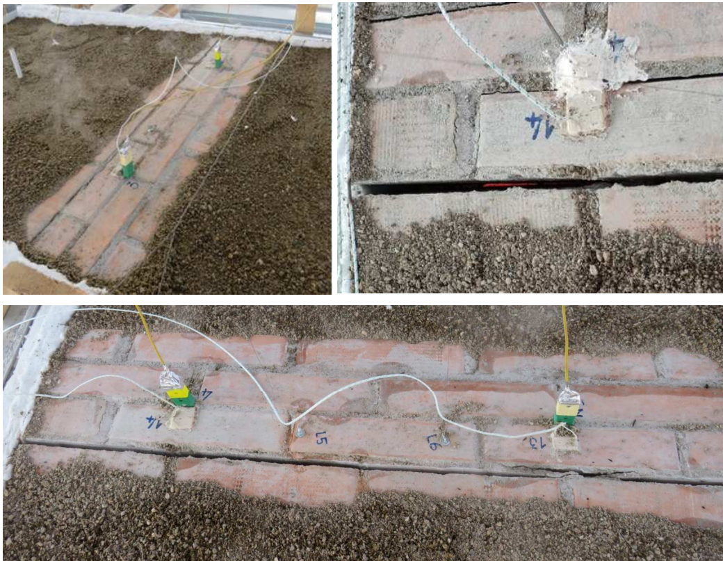
Figure 24 - Failure of brick/mortar interface and raising at the arch-crown of vault #1 during the fire exposure.
