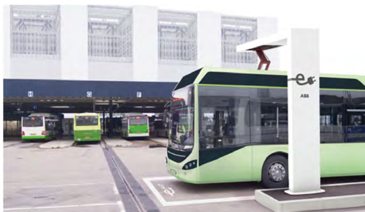
Figure 12. Volvo-ABB charging station.
