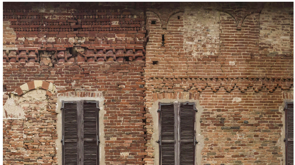
Figure 12. Section of the central part of the west front of the castle: on the left side, the earlier masonry and decorations (Period I), while on the right side, the connected masonry and Ghibelline decorations related to Period III.
