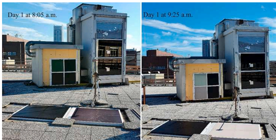
Fig. 8. Picture of the experimental set-up on the first day of the campaign, before and after the switching process.
