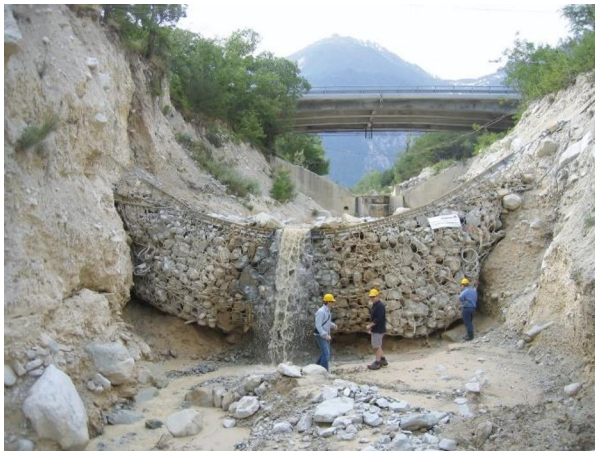
Fig. 1 Debris flow flexible barrier (Courtesy of Geobrugg Italia)
