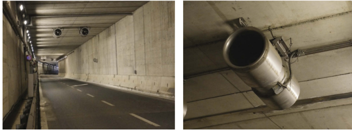
Figure 3. Jet fans positioned in pairs on the roof of a one-way road tunnel (left) and a detailed view of a single jet fan (right).
