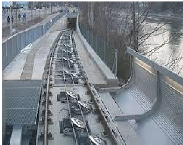
Figure 33-Picture of the rails of a funicular railway, with deflection rollers in the foreground
