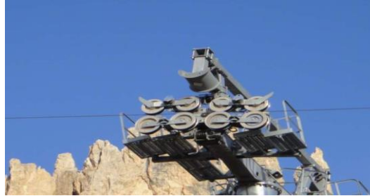
Figure 48-Picture of a support-compression tower
