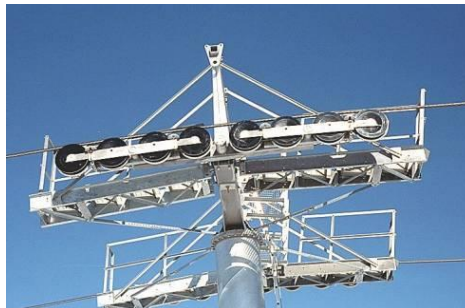
Figure 47-Picture of a support tower
