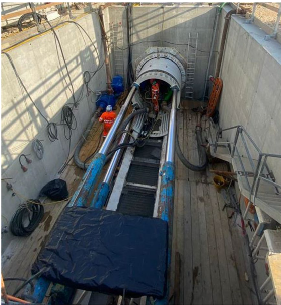
Fig. 2 The system of pushing the elements of the reinforced concrete pipeline through hydraulic jacks that contrast on the side walls of the thrust shaft
