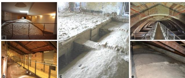
Figure 3. a) Venaria, Extrados of the vault, accessible; b) Casale, S. Evasio Cathedral archaeological path ( www.vitacasalese.it ); c) Venaria, extrados and construction phases under preservation, ground floor, invisible; d) Venaria, extrados of Galleria Grande , accessible only for maintenance activities; e) Venaria, extrados of Rimessa , not accessible.
