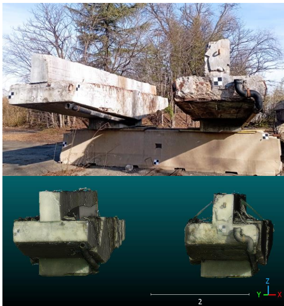
Figure 1. Up: photo of the studied beams. Bottom: TLS-generated point clouds of the studied beams.
