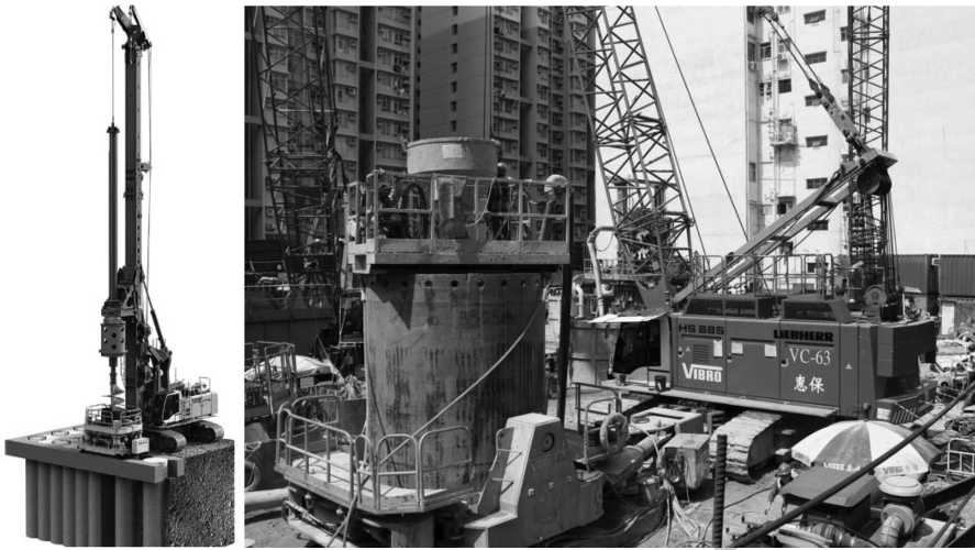
Figure 2.150 Use of casing oscillator for a secant pile job in Kelly (a) and grab (b) system.
