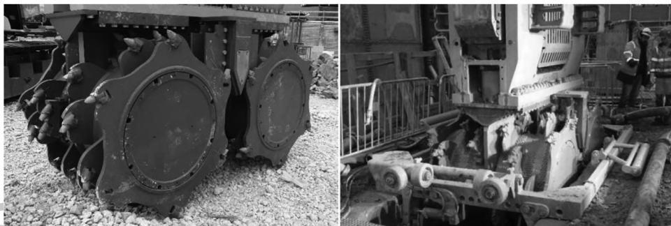
Figure 2.144 Trench cutter excavation and wall construction process - guide frame and cutter wheels. (Courtesy of Liebherr.)
