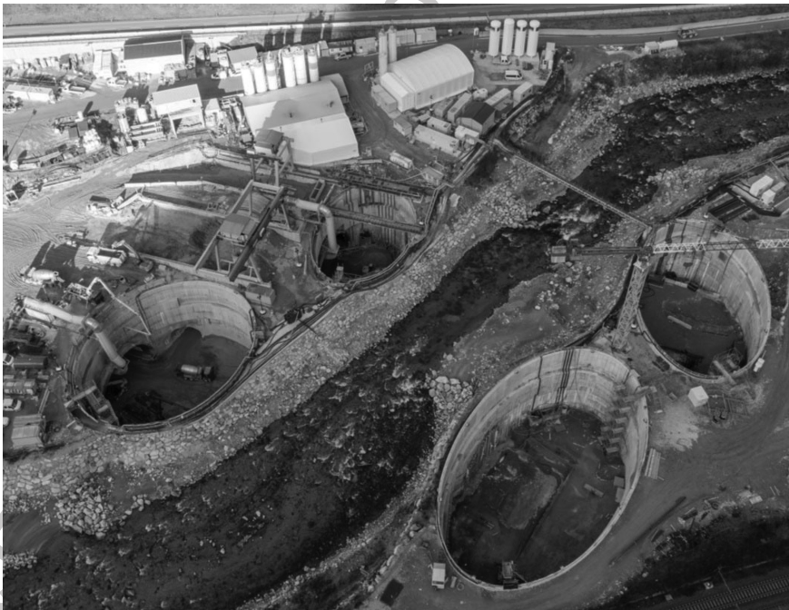
Figure 2.125 Picture of the construction phase of the four shafts near the Isarco River. (Courtesy of BBT SE.)
