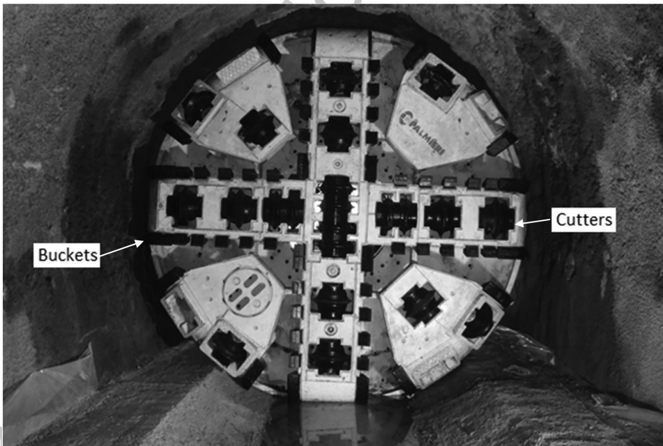
Figure 2.31 Front loading type cutterhead adopted for the excavation of a tunnel in variable conditions through soft Siltstone and hard and abrasive gneiss in Algeria.
