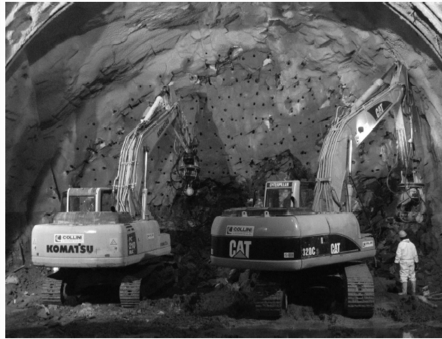
Figure 2.21 Example of a drill and split tunnel face with two machines work in parallel.
