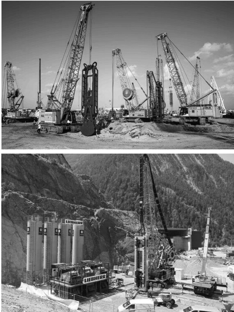
Figure 2.140 Grab excavation in port said and trench cutter in a mountains side.
