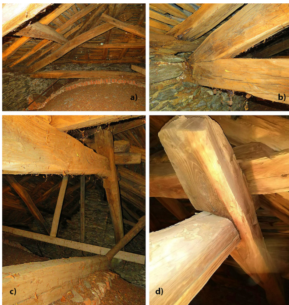
Fig. 5. (a) North truss; (b) detail of the tie beam-rafters connection, in evident degradation inside the masonry support; (c) tie beam rests on the extrados of the vaults; (d) detail of a half-lap coupling connection.
