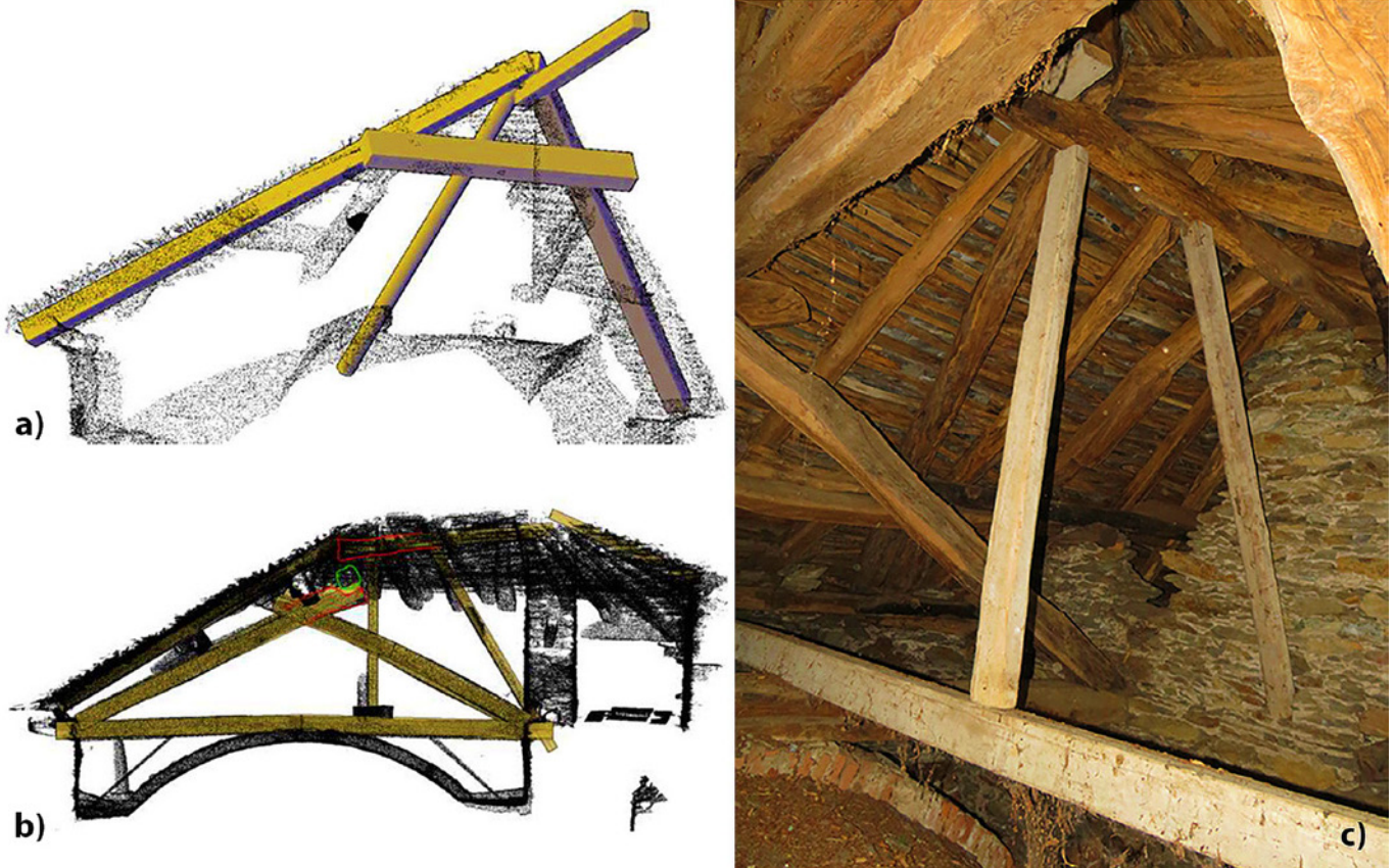
Fig. 6. (a) Laser scanner survey of the roof area, including the two cantonal beams; (b) hypothesis of the original configuration of the ridge beam; (c) props to support the ridge beam.
