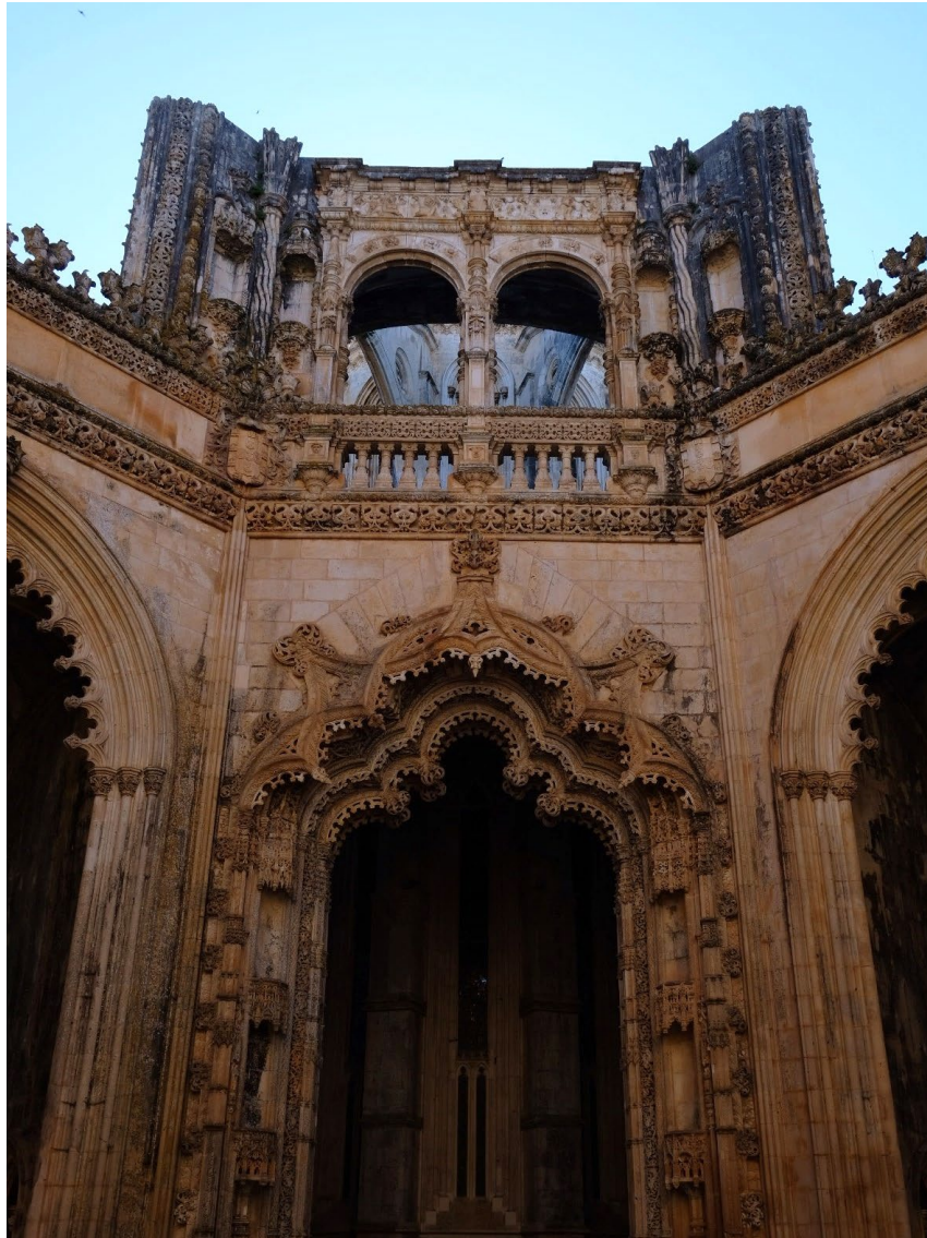
Figure 2.1. Facade and ornaments with orange patina at the Imperfect Chapel, Batalha Monastery
