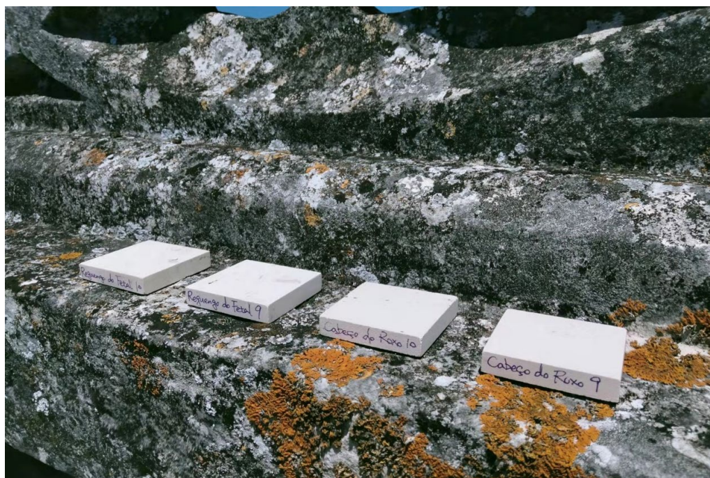
Figure 6.3. Sample tablets placed on the monastery roof (from left to right, the 1 st and 3 rd are deposited with SiO x film, the 2 nd and 4 th are uncoated).
