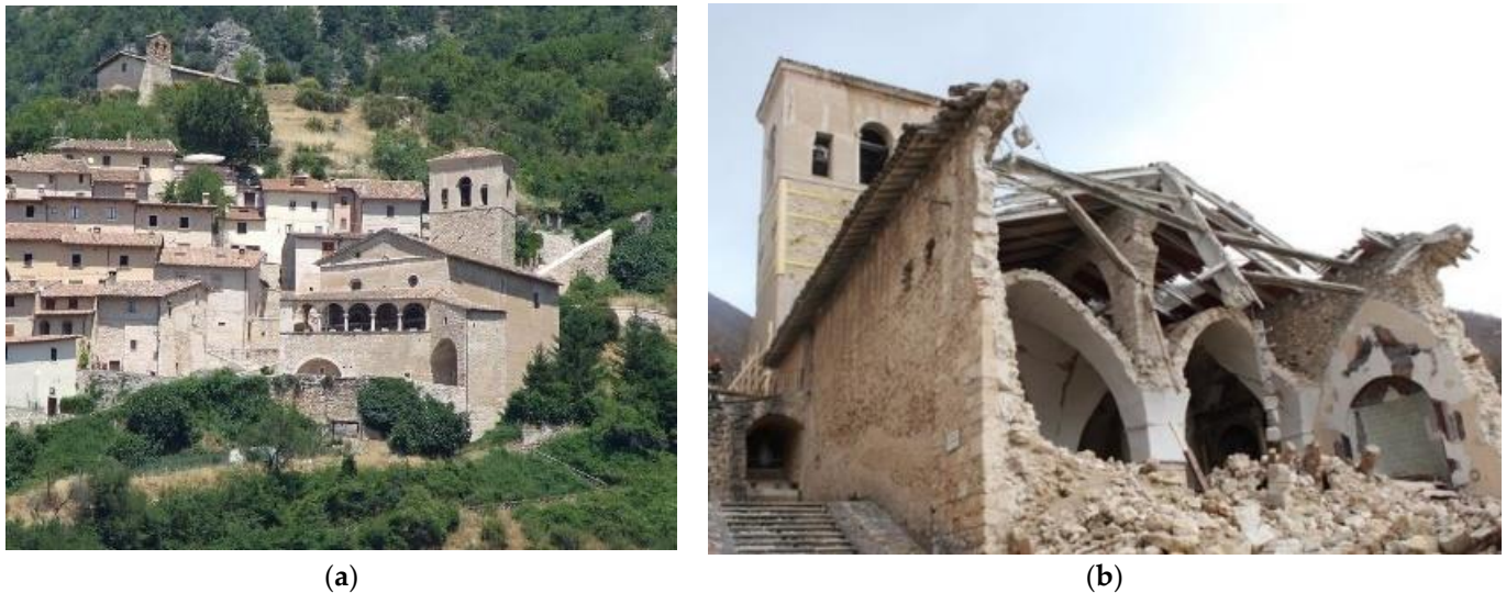
Figure 3. (a) The church of Sant'Andrea, with its bell tower and portico, prior to the 2016 earthquake. (b) The church following the collapses related to the 2016 earthquake.
