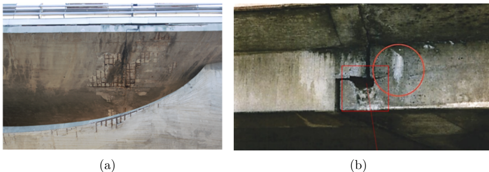
Figure 1: (a) Detail of the deterioration of the half-joint in the Musmeci bridge [13]. (b) Deterioration of the half-joint due to corrosion before collapse, [14].
