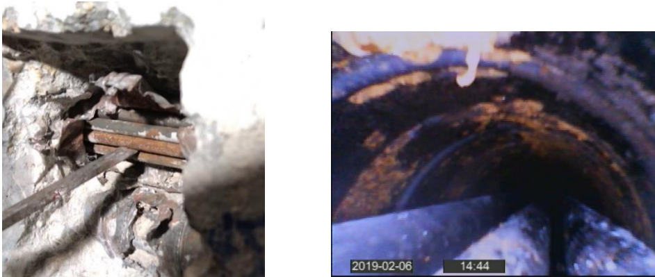
Figure 71: Visual inspection of post-tensioning tendons in the ribs (left), and endoscopy inspection inside a duct of the rib (right) (MASTRLAB DISEG, 2019)
