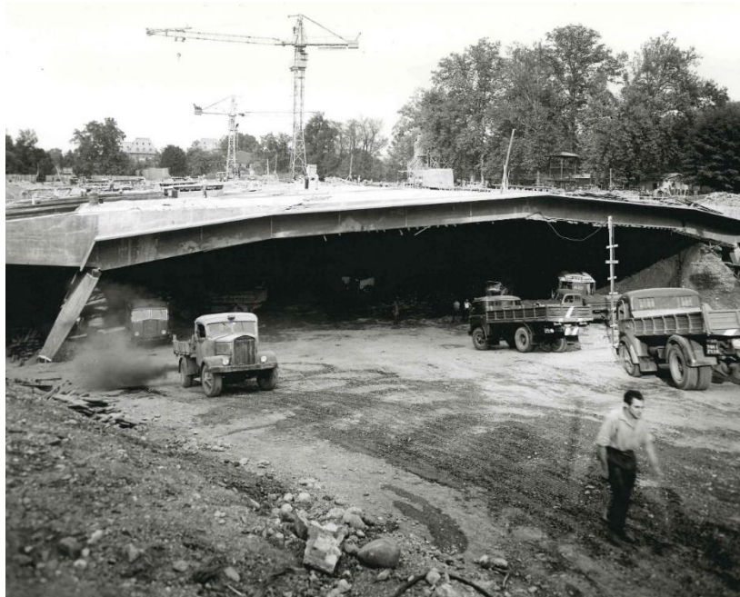
Figure 60: View of the construction site of Pavilion V of Turin Exhibition Center, 1959
