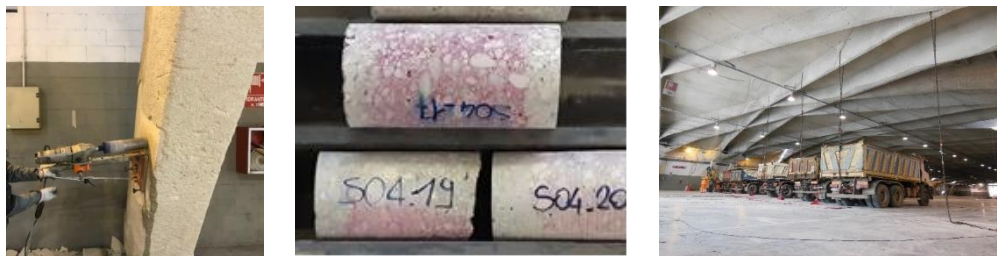
Figure 66: Pavilion V: Extraction of a concrete sample from a longer strut beam (left); carbonation tests on the samples of the ribs (center); view of the static tests with trucks connected to the ribs through jacks (right) (MASTRLAB DISEG, 2019)
