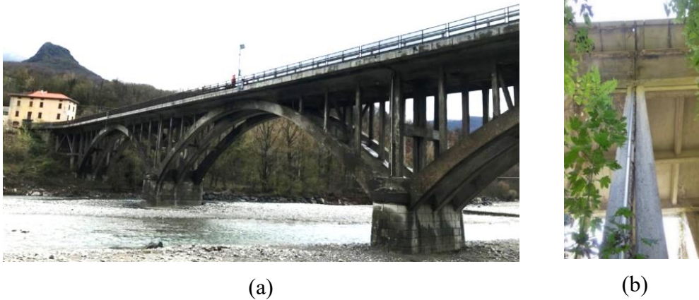
Figure 23: Lamberti bridge over the Ceno river (a); joint connecting two spans (b)
