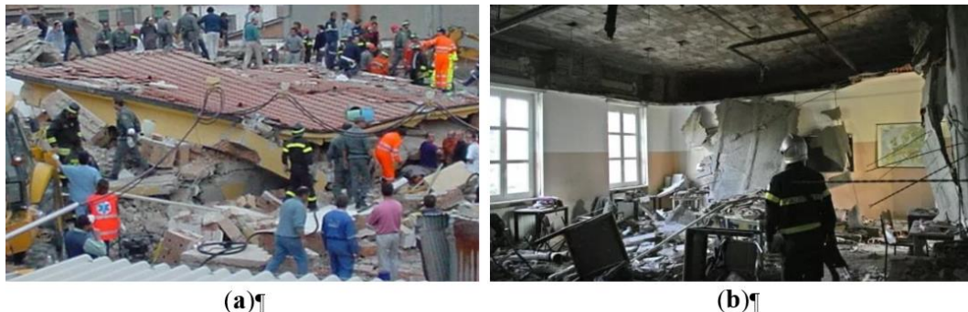
Fig. 18: Some school collapses in Italy: (a) " Francesco Iovine " Primary School in San Giuliano di Puglia [77]; (b) " Darwin " High School in Rivoli [78].
