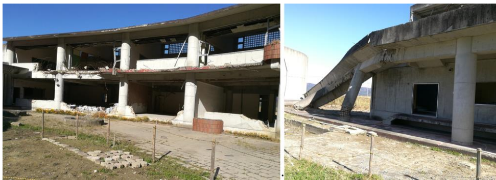
Fig. 11: Okawa Elementary school after being damaged by 2011 tsunami.
