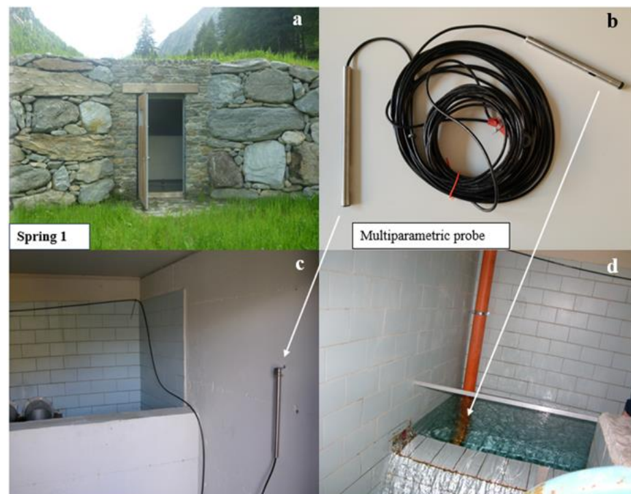
Figure 3. Mascognaz 1 spring's structure and set up: (a) External view of the spring water intake structure; (b) Multiparametric probe geometry; (c) Installation of probe data logger; (d) Installation of recording probe.
