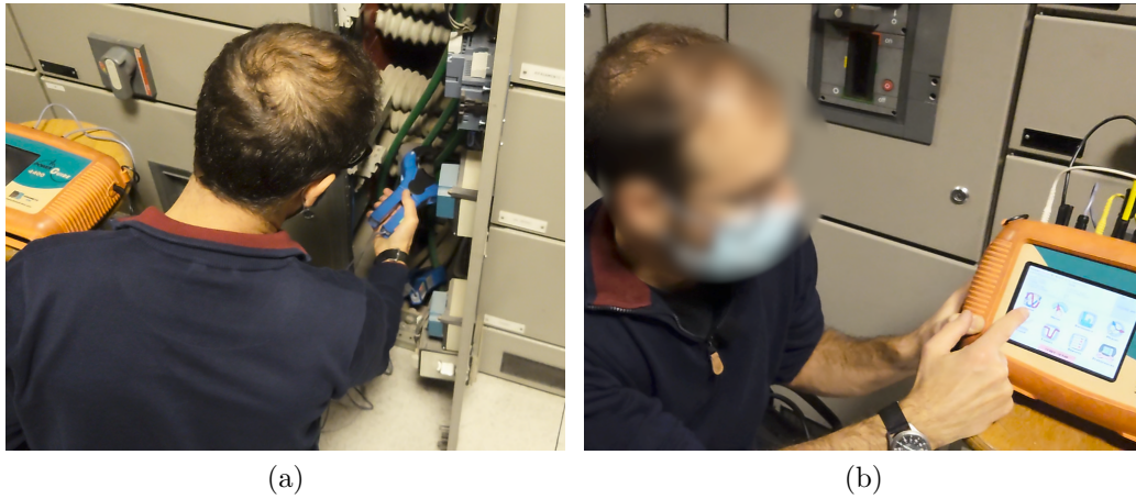
Figure 1: Details of the measuring activity: an operator (a) connects the probes to the electrical switchboard, and (b) configures the measuring instrument.
