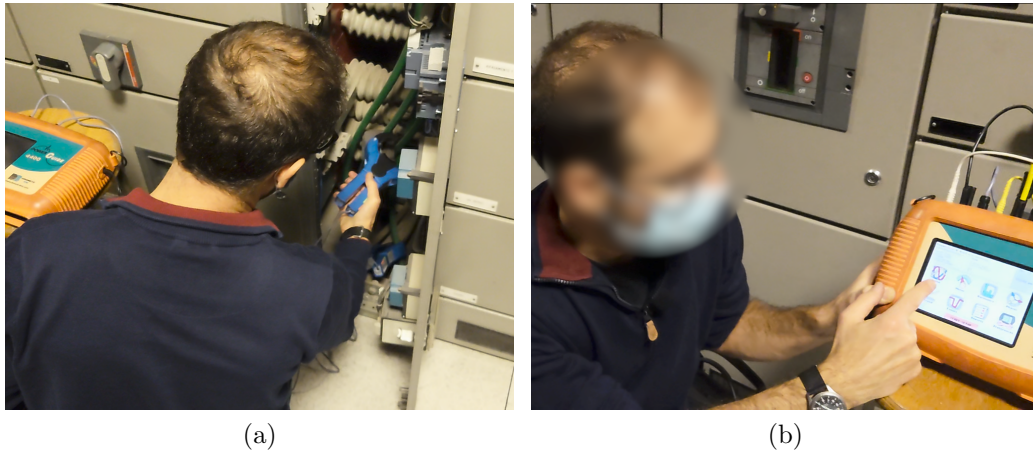
Figure 1: Details of the measuring activity: an operator (a) connects the probes to the electrical switchboard, and (b) configures the measuring instrument.
