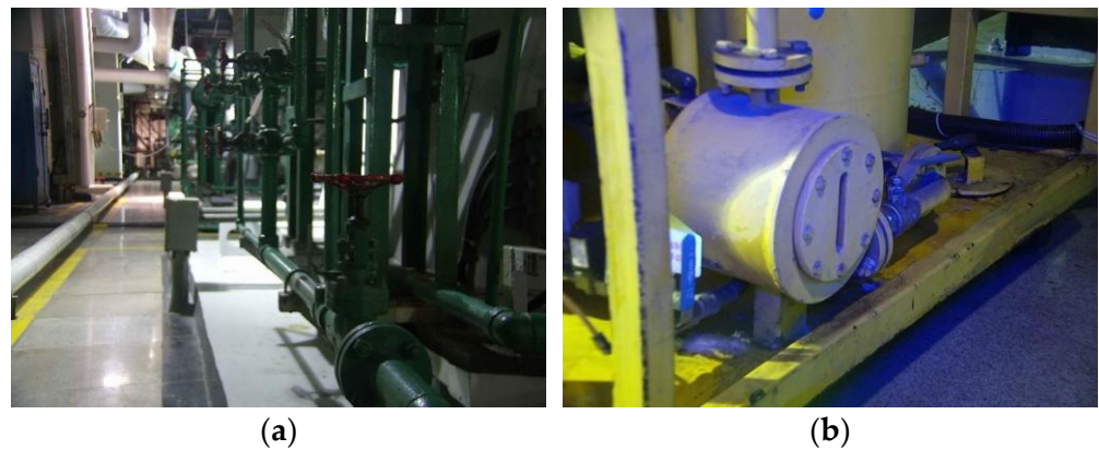
Figure 2. Significant difficulties in the actual factory environment: (a) Complex pipework layout; (b) diverse illumination conditions and non-uniform light distribution result in highly variable detection area background.
