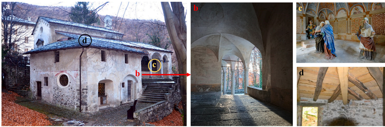
Fig. 1. The complex of Nazareth (a) with, in detail, the protective portico with starry vaults system (b), an interior view of chapel 3 “the Visitation” (c) and conservation intervention with a new angular supporting beam beneath the original secondary beams (d).
